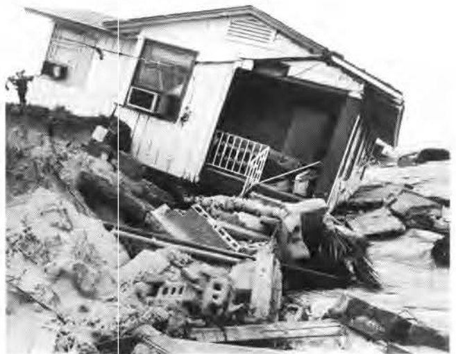
Figure 2.3. Erosion Caused This Foundation to Collapse.
