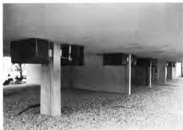
Figure 4.49. Elevated Condenser Units
